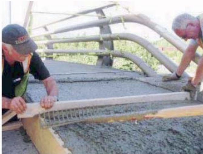
SID MILLS, left, and Gerry Monsees smooth out cement poured during the construction of wheelchair-friendly ramps on one of the two Hwy 16 bridges crossing the Skeena River.
